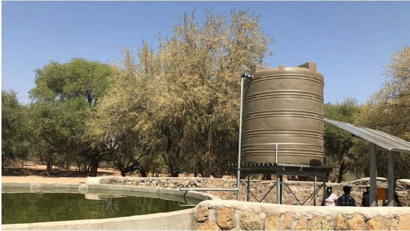
One of the rehabilitated boreholes in Kunene Region under the CBNRM EDA Project
