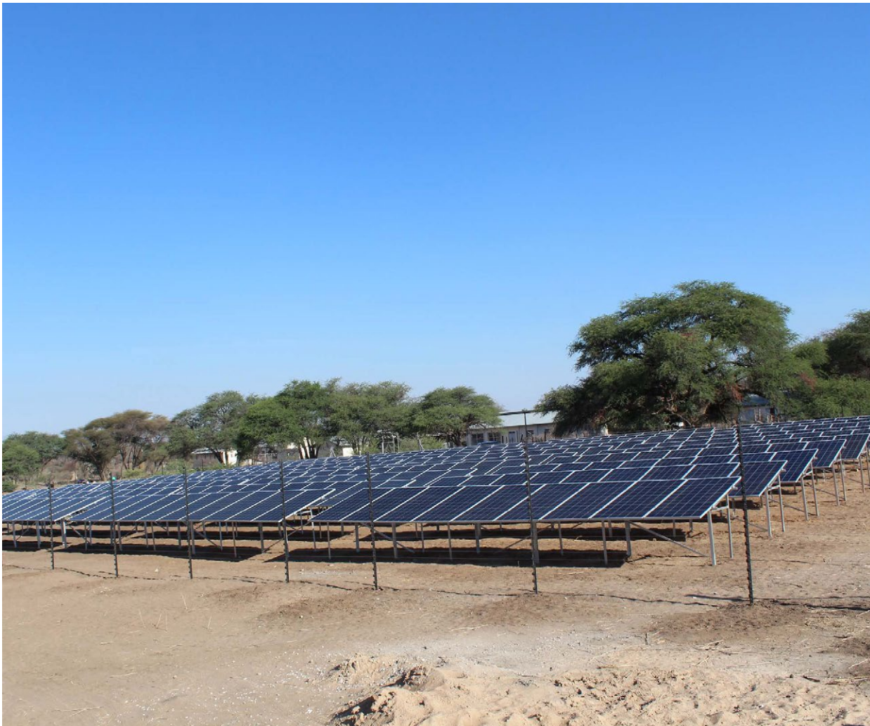
▼ Promoting use of solar energy during official handover over of 125.4Kw-PVC plant at Mashare Agricultural Development Institute (MADI) under the CRAVE Project.
